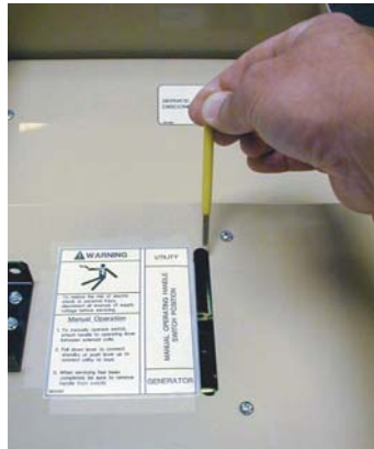
Figure 3.1 — Actuating Transfer Switch
