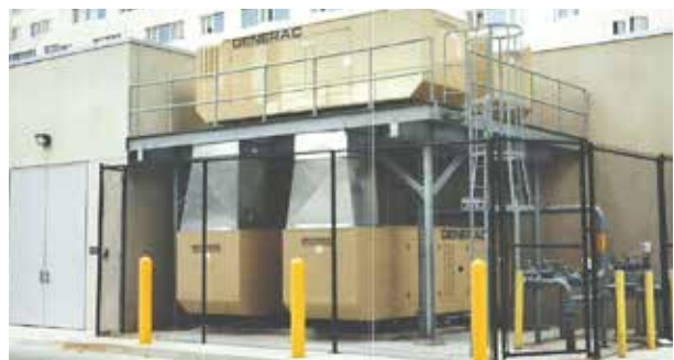
4 Generac generators stacked to meet tight footprint requirements.
