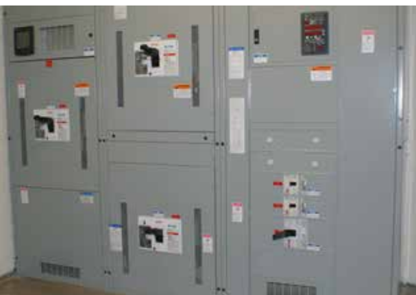
Traditional switchgear line-up with multiple generators.
